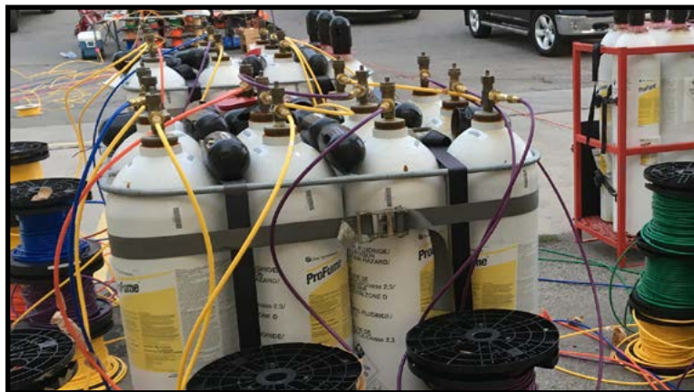
Figure 2: It is highly recommended to release fumigant from outside the building to minimize applicator exposure to the fumigant and increase safety. Here, operators get ready for a large fumigant operation with cylinders outside the structure attached to hoses leading inside. (Photo © Douglas Products).
