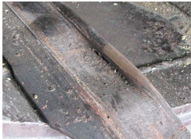
Figure 5-6. A welder certified in confined space entry would be needed to repair this broken weld on a track inside a cylinder.
