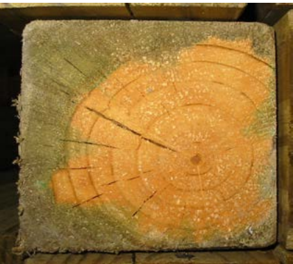
Figure 1-1. Effect of sapwood and heartwood on penetration by preservative in round utility pole (top) and sawn member (bottom). Photos: USDA Forest Products Laboratory
