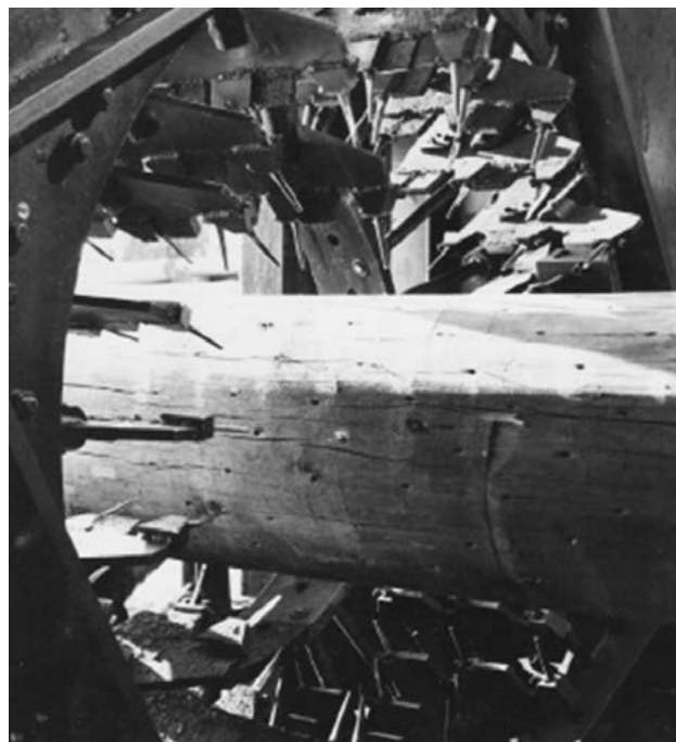
Figure 6-3. Incising permits better penetration of preservative. (Photo courtesy of USDA Forest Products Laboratory)
