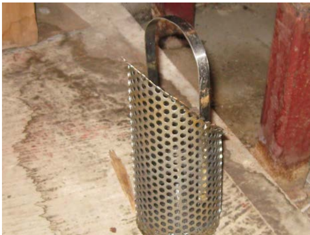
Figure 5-4. Cleaned line filter
